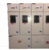
Meter Panel Board
