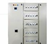
Lighting Distribution Board
